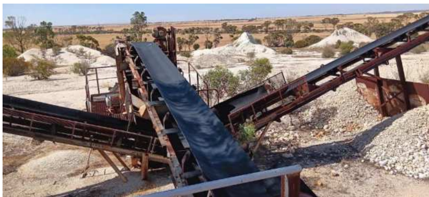
Looking east from the Mukinbudin quarry over the conveyor belts of the screening plant (Picture by Stuart Jeffries)
